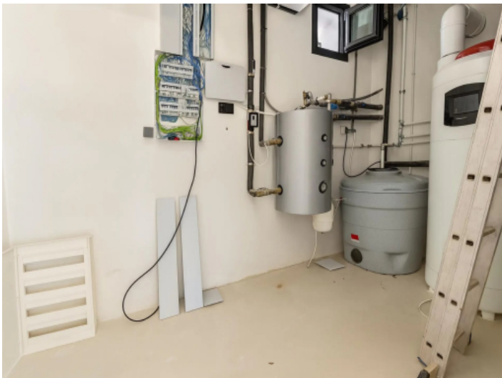
Technical room of the energy-efficient villa
