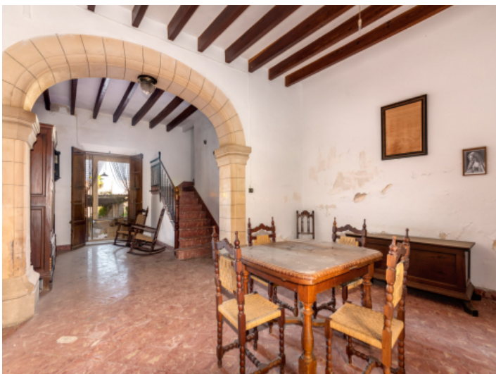
Townhouse in the centre of Son Servera with garden and terrace for reformation
