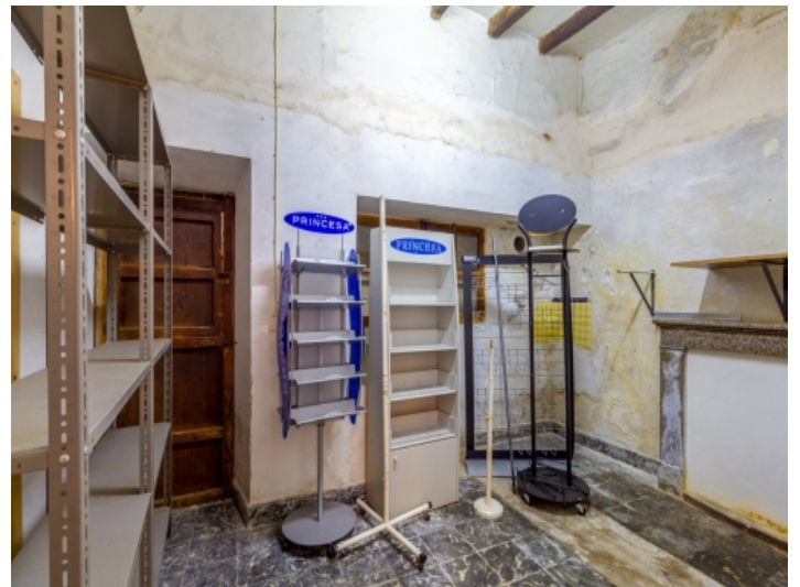
Room in need of refurbishment
