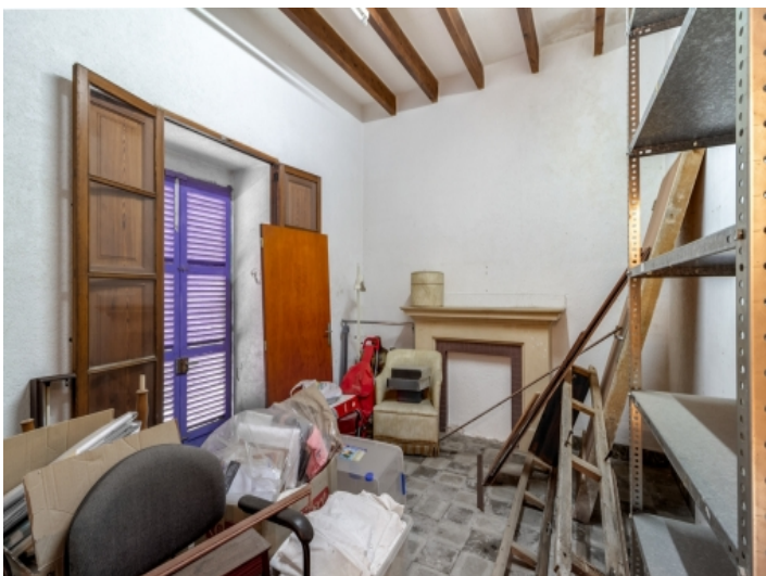
Room in need of refurbishment
