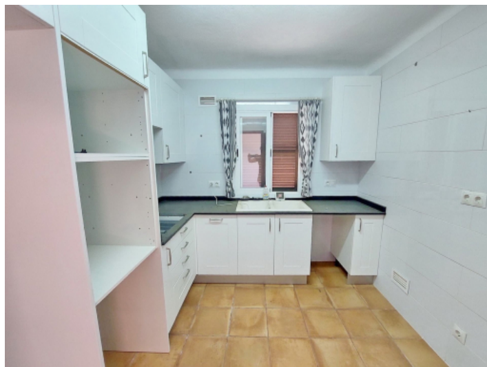
Kitchen in need of renovation
