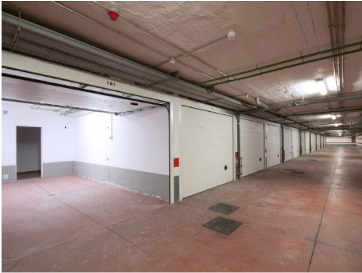
Underground parking with automatic gate
